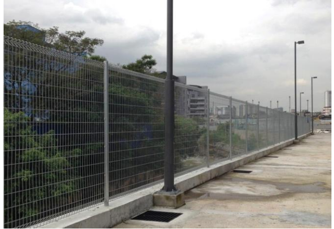
Anti Climb Perimeter Fencing
